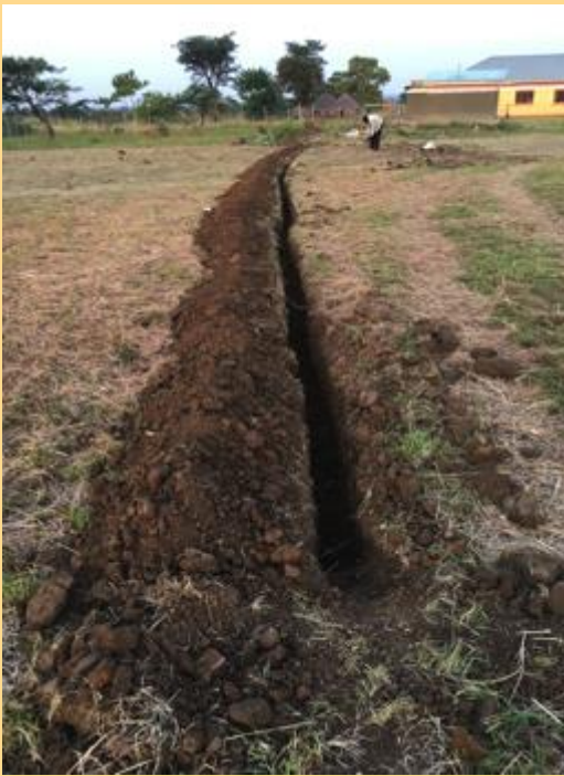
Water Piping throughout the property
