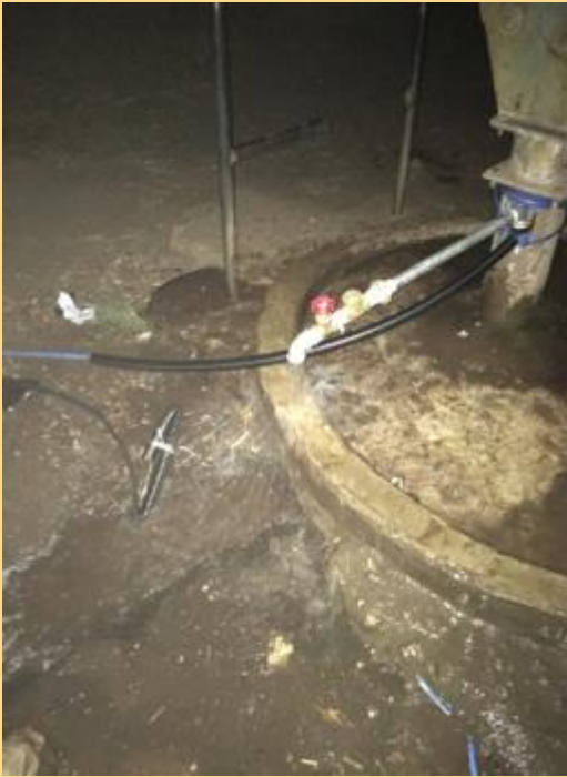
New electric well pump
